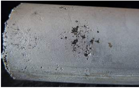
Figure 17.17 Pitting of a 316L stainless steel pipe surface by a phosphate solution. (Photograph courtesy of Rick Adler/Adler Engineering LLC of Wyoming USA)
